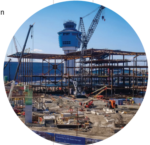
LaGuardia Gateway Partners is building a new central terminal building at LaGuardia Airport
